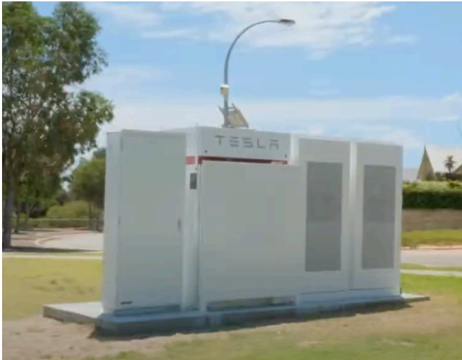
Meadow Springs, WA (Western Power)
